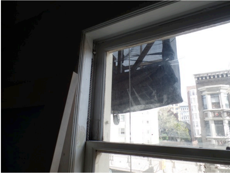
Figure 10. Overview of typical wood double-hung window unit along the north elevation. (Photograph by Garavaglia Architecture, Inc., April 2015.)
