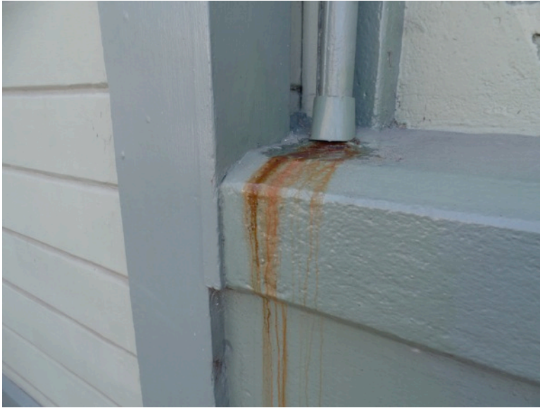
Figure 22. Corroded downspout along north elevation. (Photograph by Garavaglia Architecture, Inc., April 2015.)
