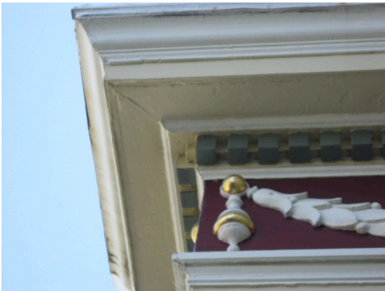
Figure 18. Peeling paint at perimeter fascia. (Photograph by Garavaglia Architecture, Inc., April 2015.)
