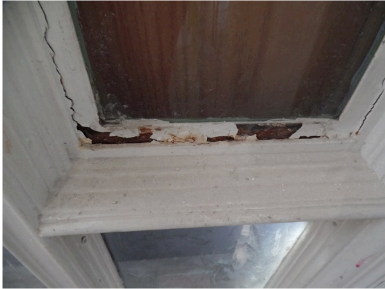
Figure 22. Peeling paint and corrosion at ground floor window. (Photograph by Garavaglia Architecture, Inc., April 2015.)
