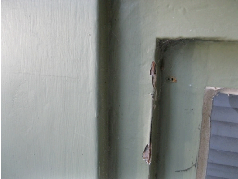
Figure 19. Peeling paint at basement level. (Photograph by Garavaglia Architecture, Inc., April 2015.)
