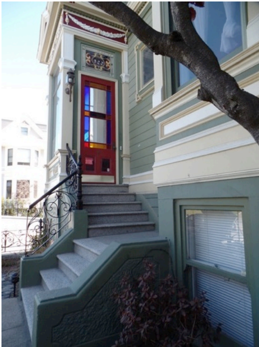
Figure 9. Detail of main entry along Steiner Street, with detail of steps and entrance portico. (Photograph by Garavaglia Architecture, Inc., April 2015.)
