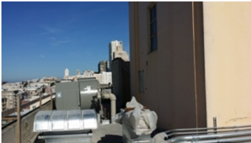
Figure 15. Overview of main roof, showing mechanical equipment and elevator bulkhead. (Photograph provided by RLJC, April 2015.)
