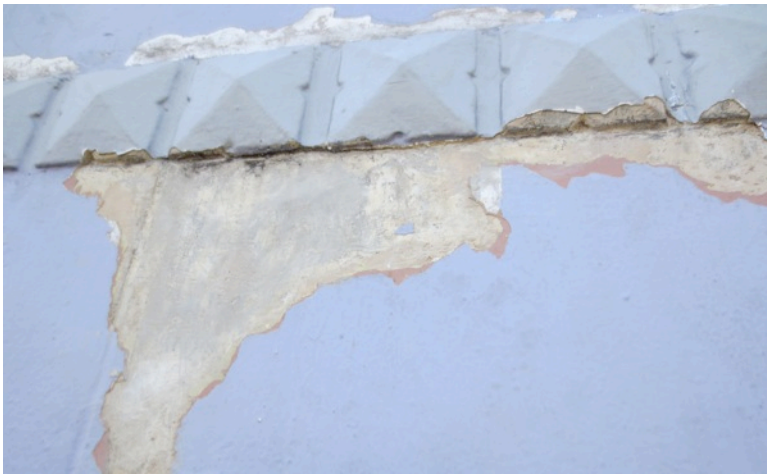
Figure 21. Peeling coating along the north elevation. (Photograph provided by RLJC, April 2015.)
