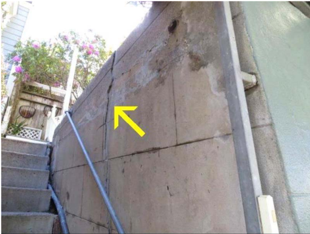
Cracked and leaning retaining wall
