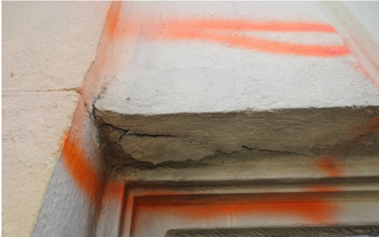
Figure 18. Cracked concrete above window at the seventh floor along the north elevation. (Photograph provided by RLJC, April 2015.)
