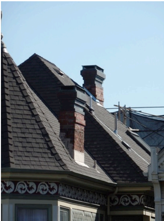
Figure 15. Detail of chimneys at south end of roof. (Photograph by Garavaglia Architecture, Inc., April 2015.)
