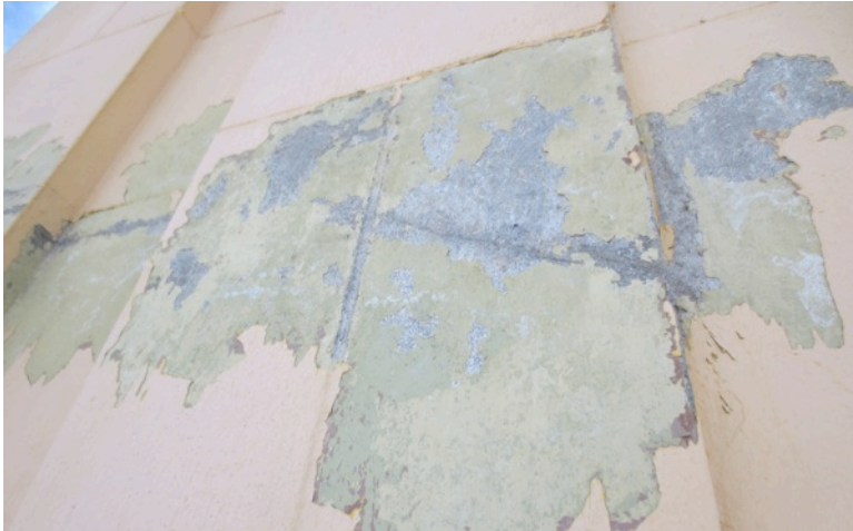
Figure 20. Peeling coating along the north elevation. (Photograph provided by RLJC, April 2015.)
